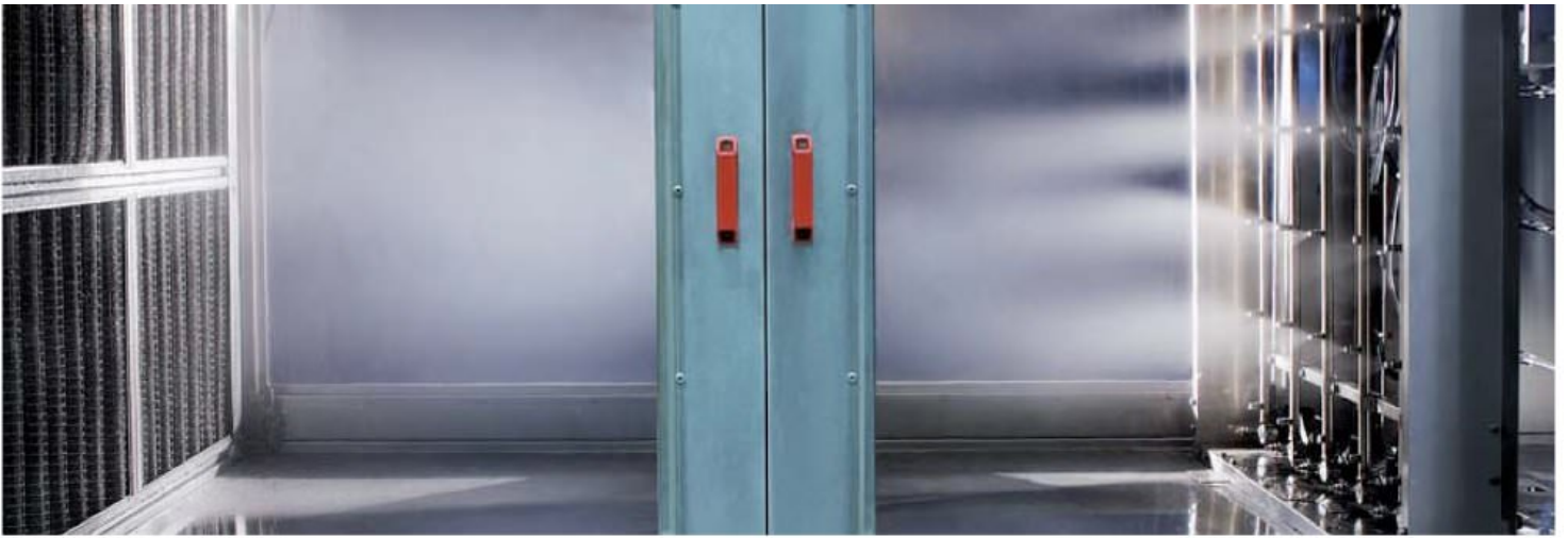
Tests in the duct performed at the CAREL labs: up to 95% of the atomized water is absorbed by the air, which is efficiently humidified and cooled, minimizing water and energy consumption.
